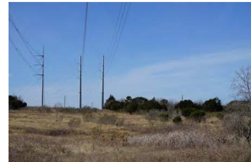
Regional overhead power lines passing through Walter E. Long park.
